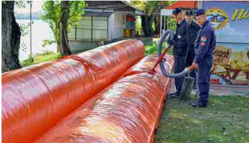
Workers securing the banks of the River Tisza in Hungary against flooding. © SDC
