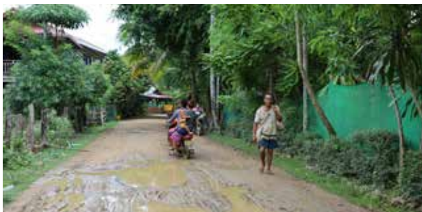
In need of repair. The 11-kilometer road between Don Khone and Don Det islands will be upgraded to an all-weather surface under the second phase of the ADF-assisted Greater Mekong Subregion Tourism Infrastructure for Inclusive Growth Project (photo by Xaykham Manilasith).
