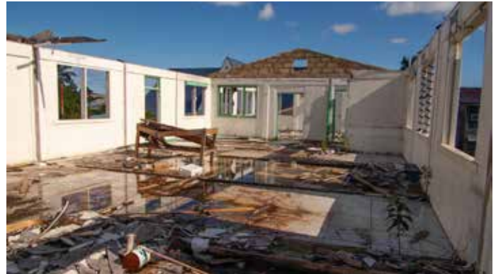
Still recovering. One year after Cyclone Gita, buildings without roofs and with other damage (above and right) are still visible across Tonga (photo by Lester Ledesma).
