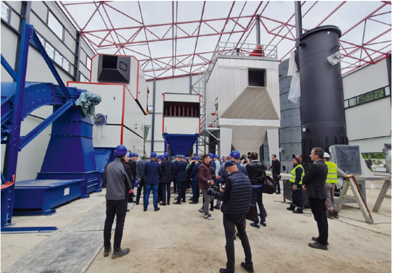
New biomass fuel plant in Priboj, which will contribute to the increase in use of renewable energy sources in Serbia to reduce pollution. Project 'Renewable Energy for District Heating Programme in Serbia'
