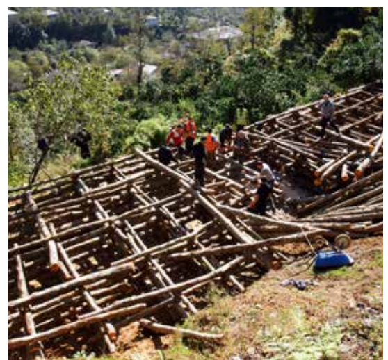
A timber crib wall has been built to ensure safe passage for residents of Joko, Ajara. Previously people relied on a narrow, unpaved road on a landslide-prone slope.
