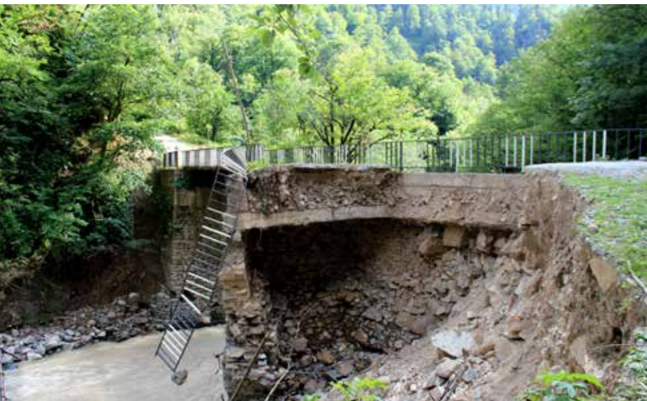
This bridge in Ajara was destroyed by a flood. Natural disasters like floods destroy local infrastructure, cutting off rural villages from their markets and destroying fields. Protective measures aim at reducing damages to riverbank farms.
