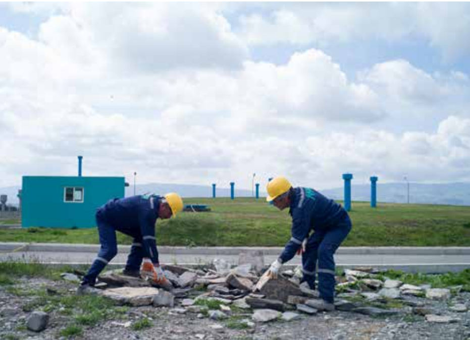
With the rehabilitation and construction of water infrastructure, rural populations in Azerbaijan now have access to potable water on a regular basis.
