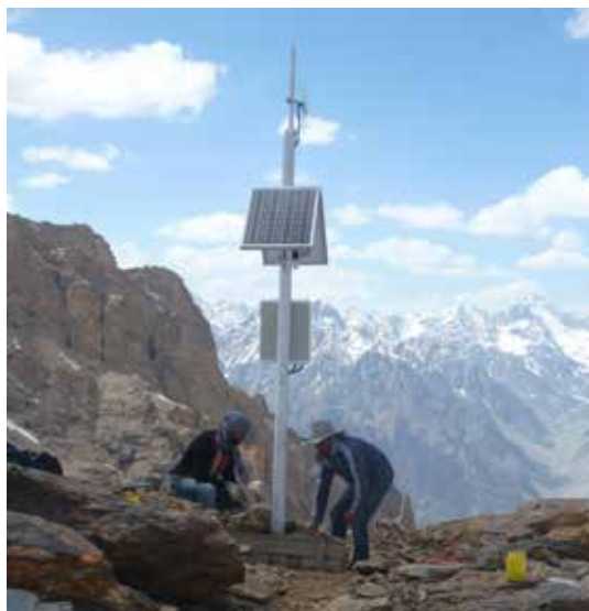
Installation of early warning system in Shugnan district, Tajikistan. © FOCUS Tajikistan
