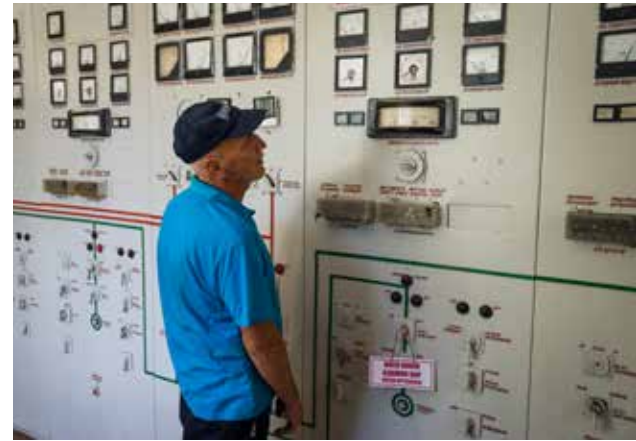
Khorog HPP Dispatch Electric Panel, Tajikistan. © Pamir Energy
